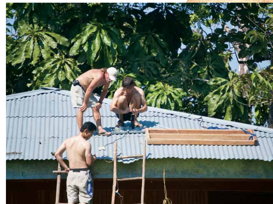
Future Scientist members Tyson Kim, Bob Pollard, and Richard Novak install solar panel framing on the roof of the orphanage director's house. The panels now power a laptop and TV and reduce usage of a gas-powered generator.
